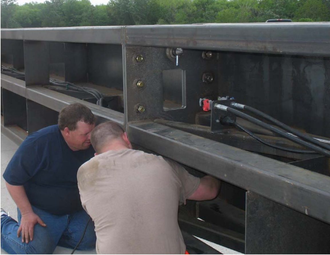
Figure 2.5 – Wall Panel Being Attached to another Wall Panel with Twelve Bolts (Unconnected Hydraulic and Electrical Lines are Also Shown)
